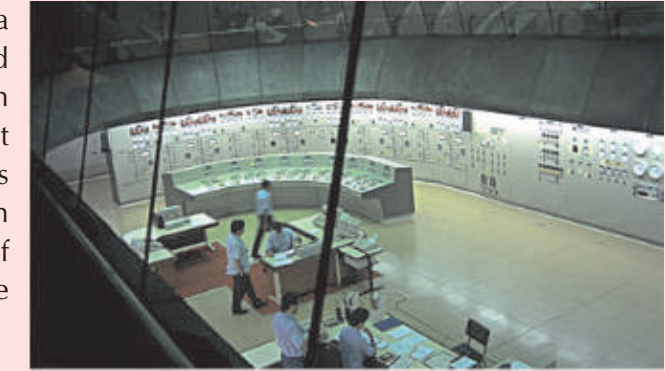
The control center of the 18 generators. Left half of it (in Brazil) controls the 60 Hz units, right half (in Paraguay) controls the 50 Hz units
